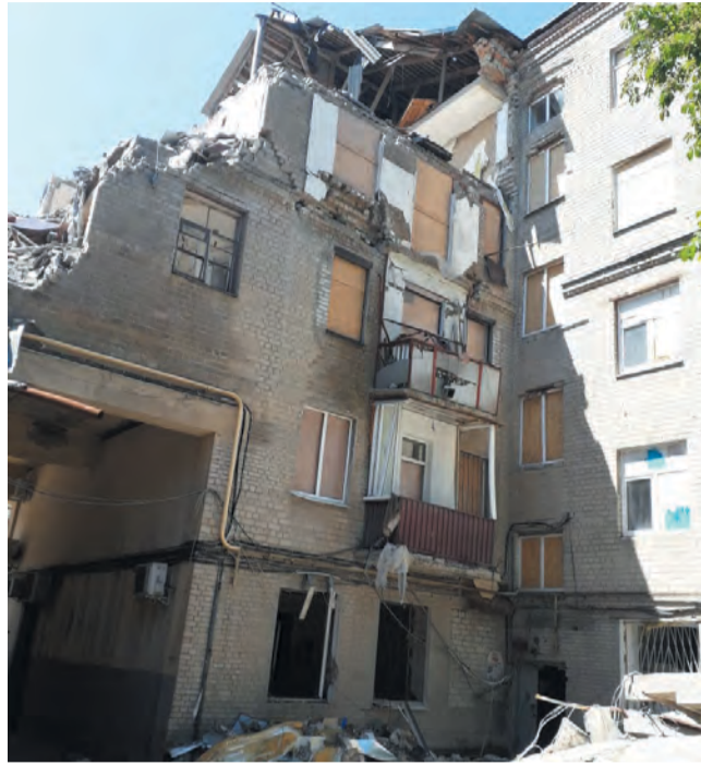
The destroyed apartment building in Kharkiv. Photos: C4I
